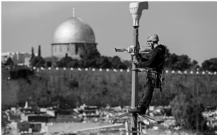
An Israeli technician installs a surveillance camera in Ras al-Amud, a neighborhood southeast of the Old City in occupied East Jerusalem, as part of a project to widen surveillance in the city. Under this project, over 750 surveillance cameras are being installed throughout the Old City and Jerusalem's Palestinian neighborhoods. (24 January, Ahmad Gharabli/AFP/Getty Images)
